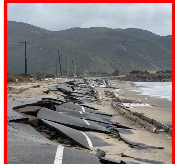
Beach Rd east bound lane undercut and collapsed
